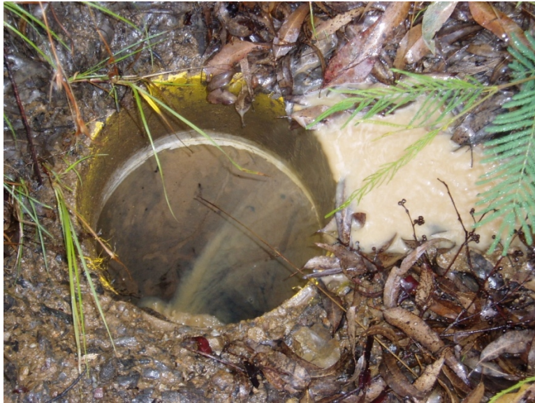
Fig. 5. 'Elbow' relief pipe inlet conveying sediment-laden water, Kangaroo River State forest
