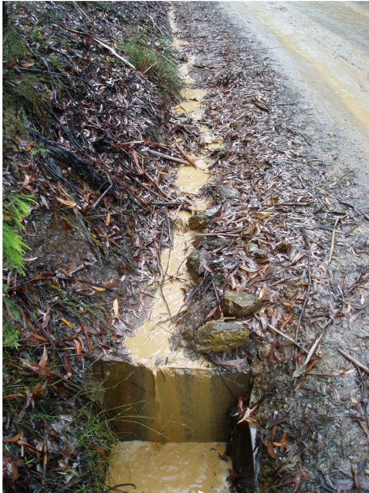
Fig. 4. Sump relief pipe inlet on Black Mountain Road, Kangaroo River State forest conveying sediment-laden water from the table drain during a rain storm. The arrow shows the direction of flow in the pipe beneath the road surface
